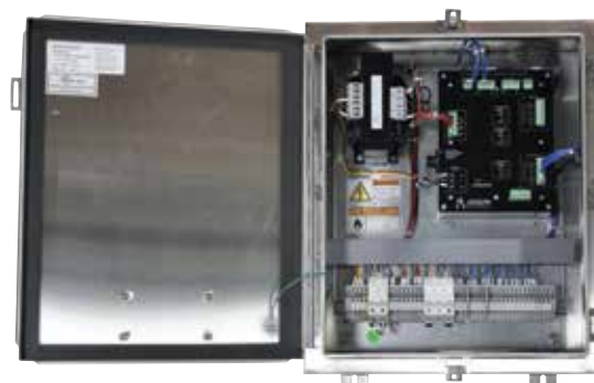
Motor Control Unit
